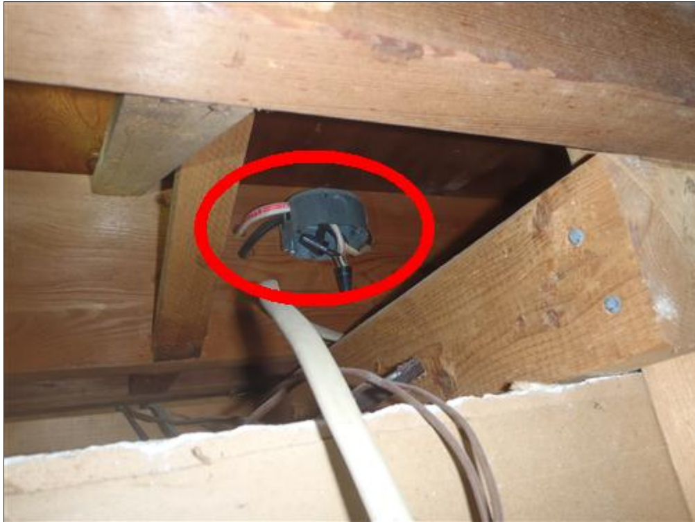
7.3 Picture 1 Open junction box
