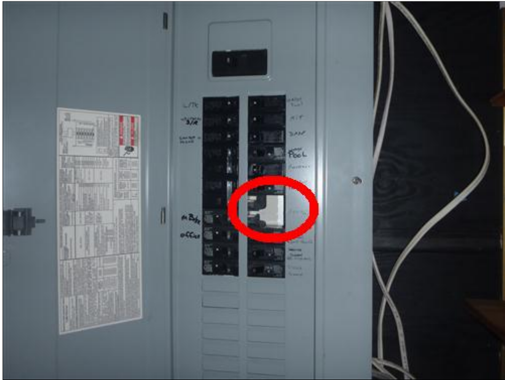
7.1 Picture 1 Missing knock out
