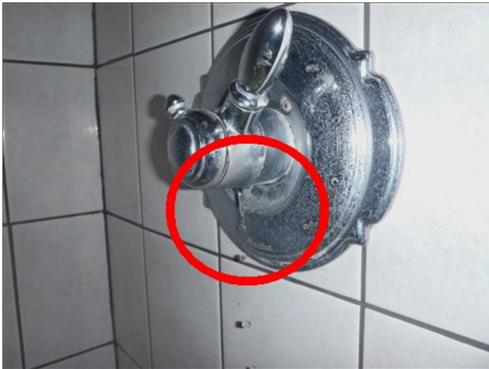
6.1 Picture 2 Leaking valve
