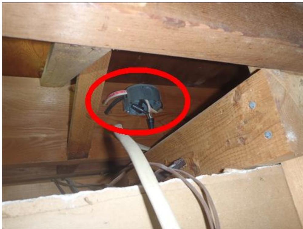
7.3 Picture 1 Open junction box
