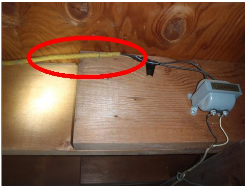
7.2 Picture 1 Damaged wire
