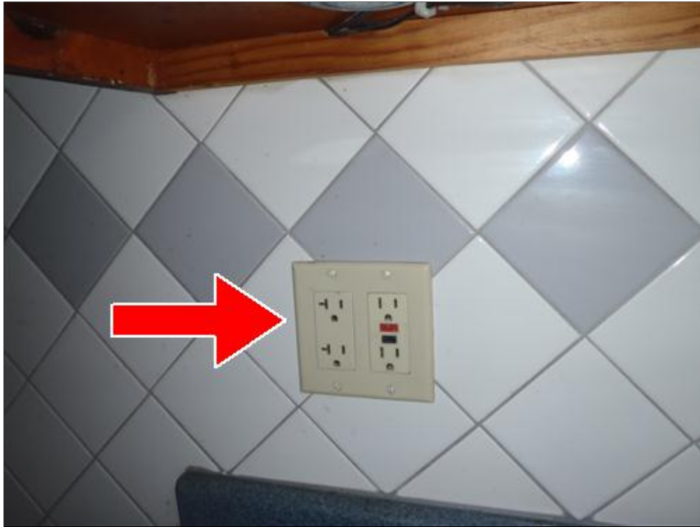
7.4 Picture 1 Not GFCI protected
