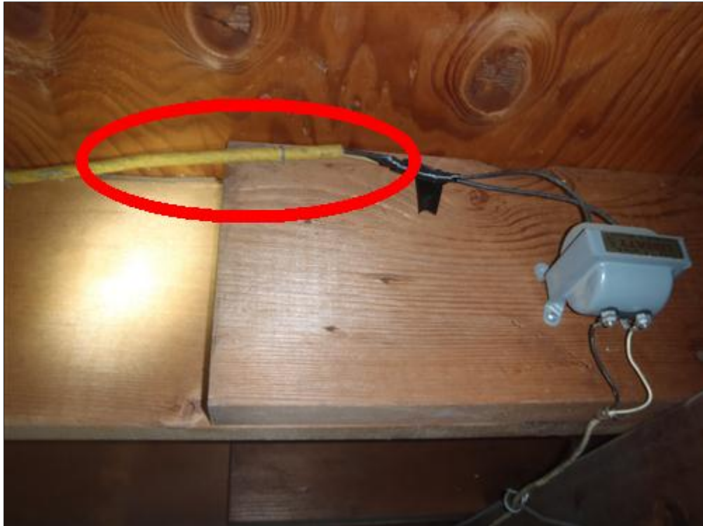
7.2 Picture 1 Damaged wire
