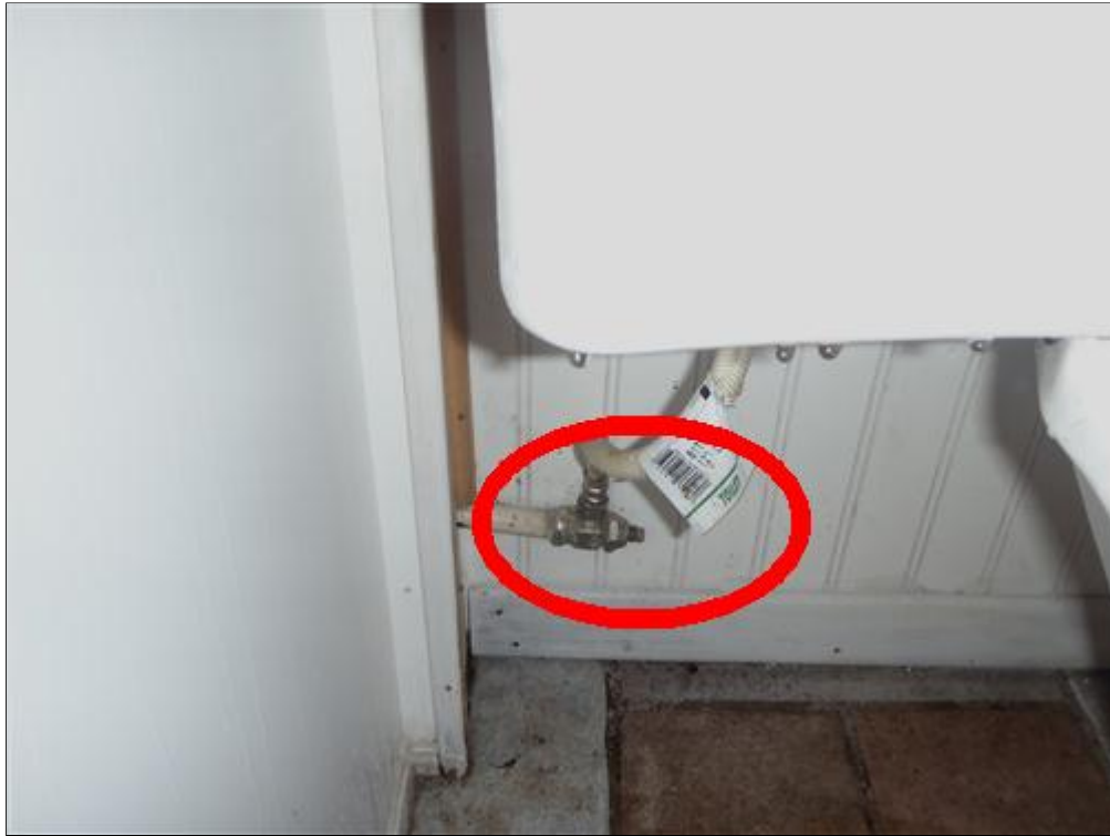
6.1 Picture 5 Missing valve
