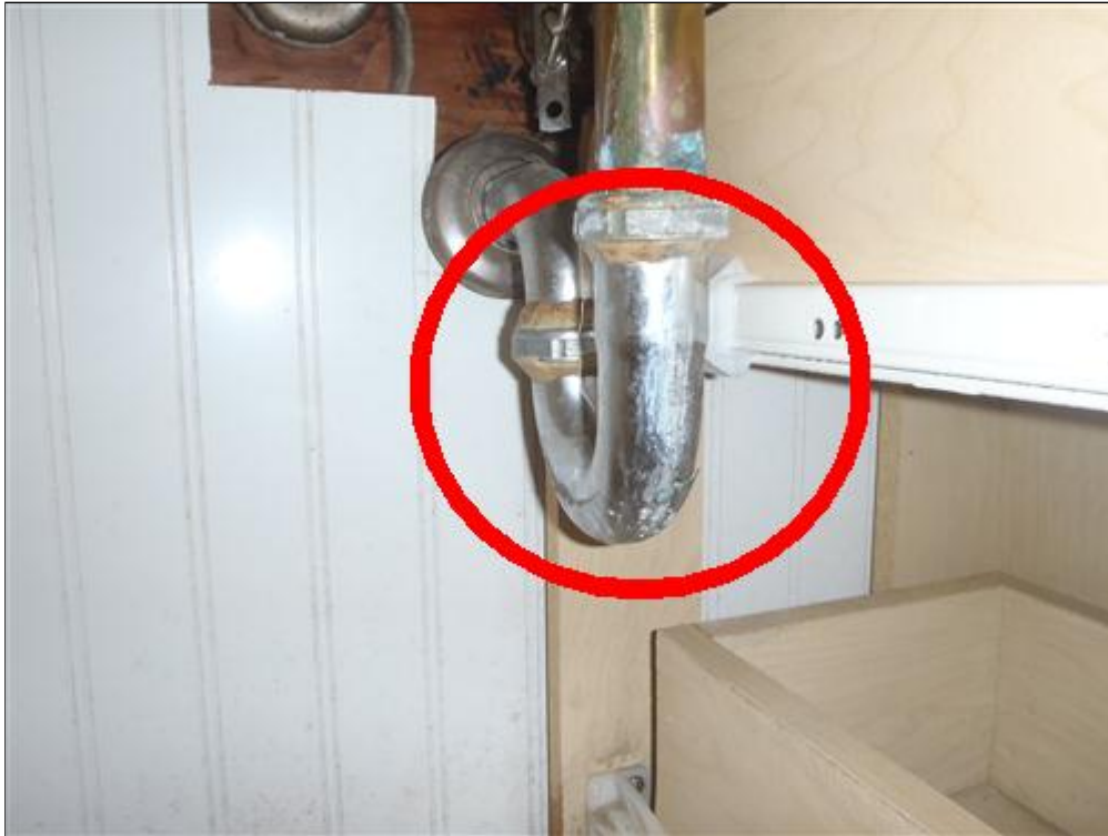
6.1 Picture 1 Waste trap
