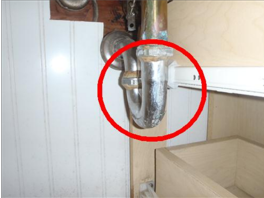
6.1 Picture 1 Waste trap
