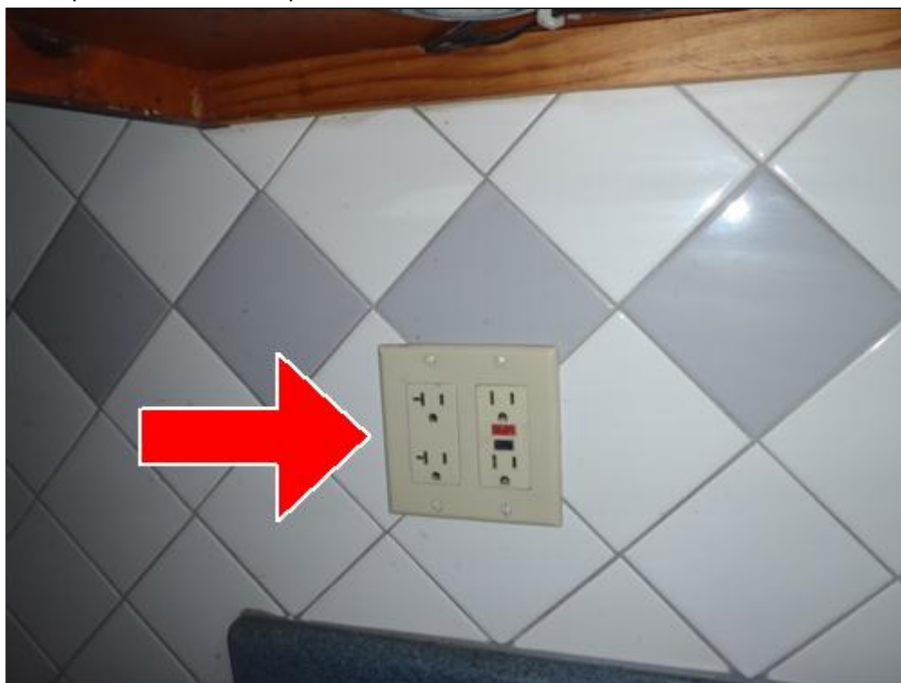
7.5 Picture 1 Kitchen GFCi
