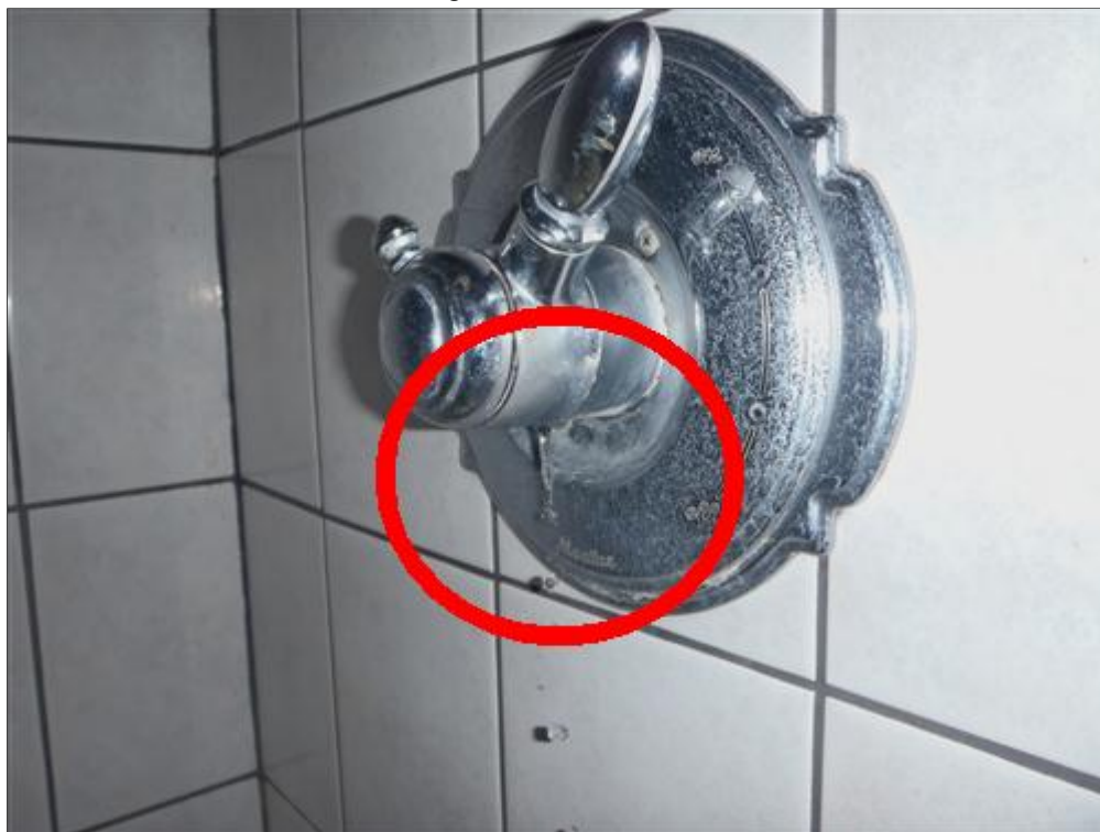
6.1 Picture 2 Leaking valve
