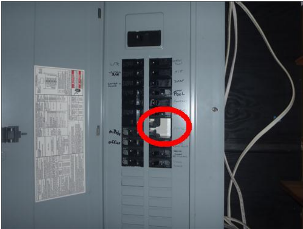
7.1 Picture 1 Missing knock out
