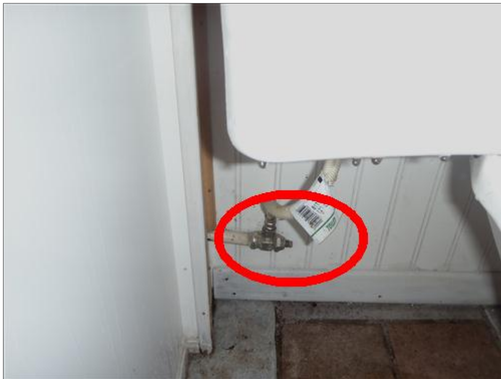
6.1 Picture 5 Missing valve
