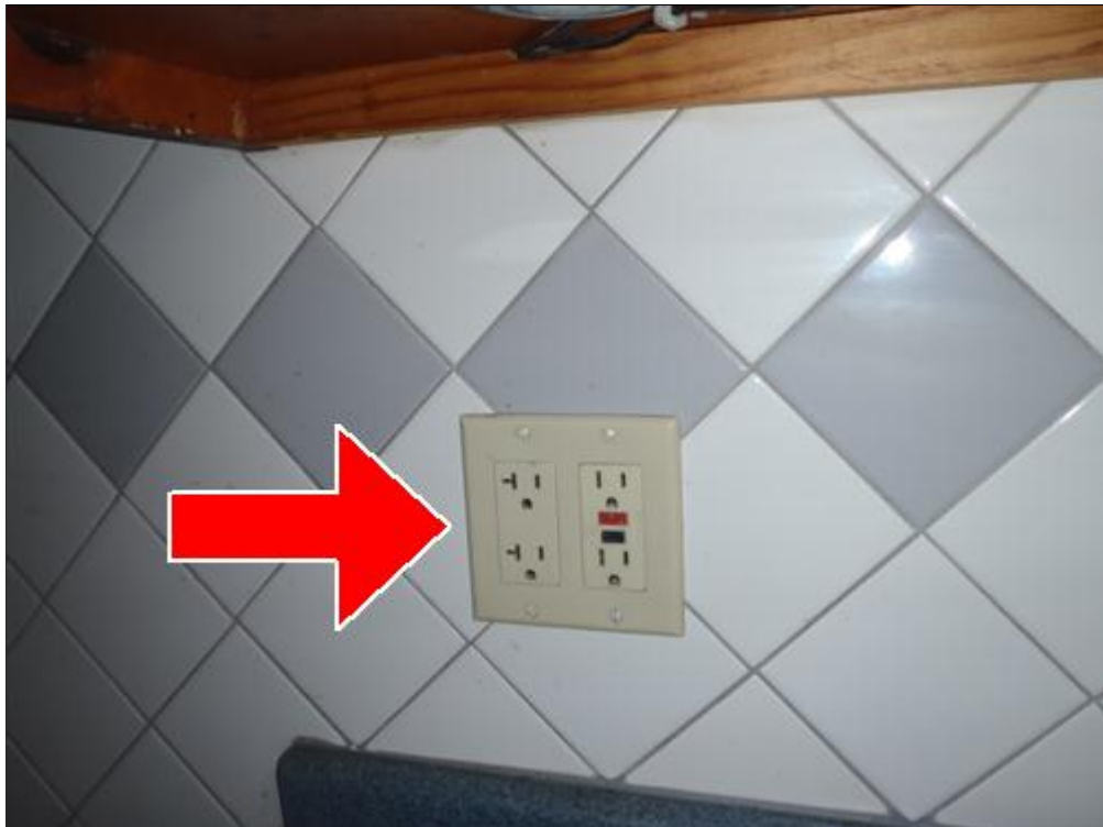
7.5 Picture 1 Kitchen GFCi
