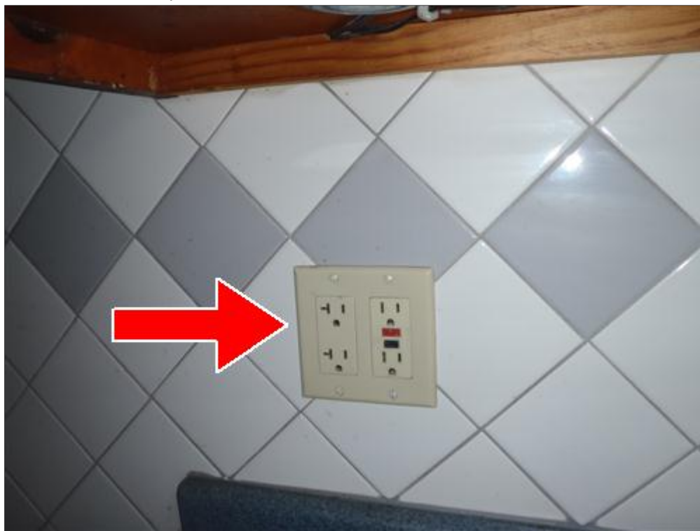
7.4 Picture 1 Not GFCI protected
